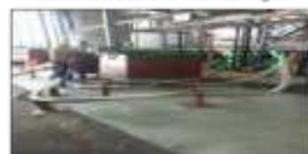
Hanging of Flexible pipes for ease of cleaning
